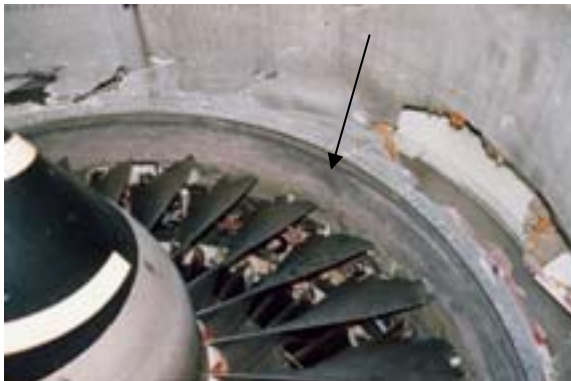
Fig. 5. View of the fan containment shroud showing the released blade impact point.
