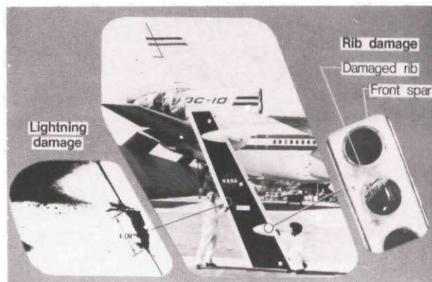
Figure 11. DC-10 graphite/epoxy rudder damage.
