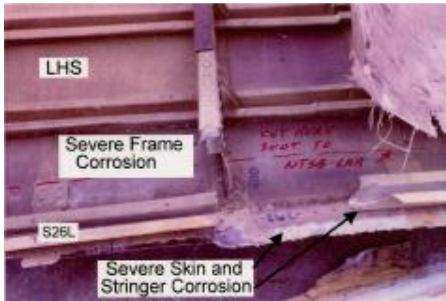
Figure D6: Photo Illustrating Loss of Frame and Stringer Due to Severe Corrosion
